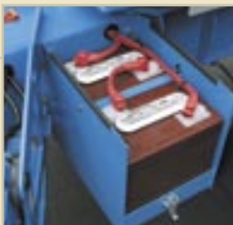
EASY ACCESS TO BATTERIES
