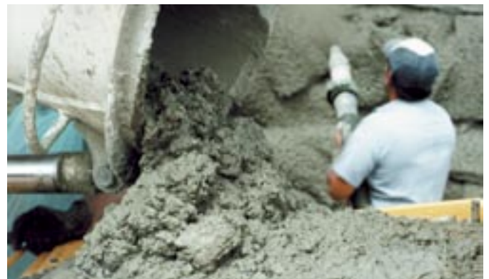
High volume shotcreting (wet gunning) with the adaptable LS-40 is all in a day's work for this versatile concrete pump.
