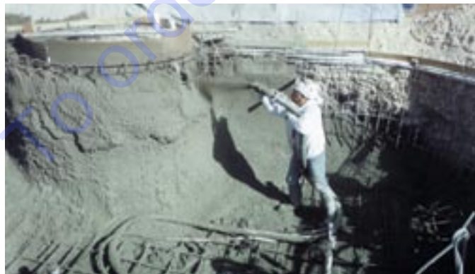
The LS-50, with its powerful ability to handle the toughest shotcrete mixes, enables a swimming pool contractor to apply shotcrete to two pools a day.
