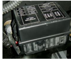
Fuse Box & Relays
