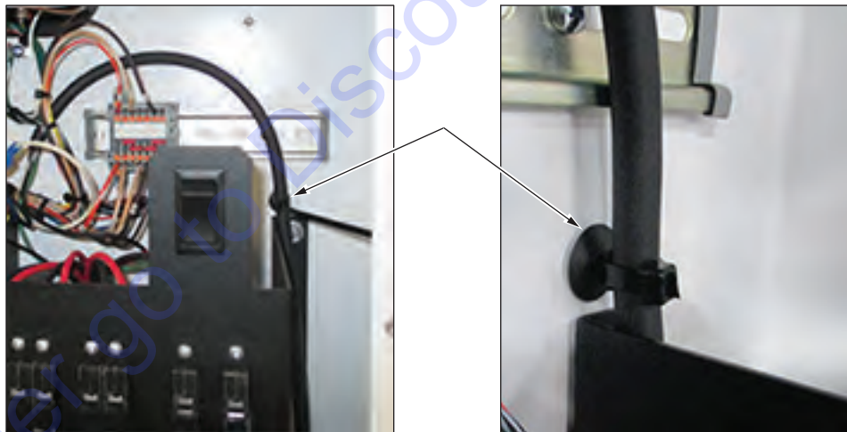
Figure 26 - Heater Harness, Secured to Cable-Tie Mount
