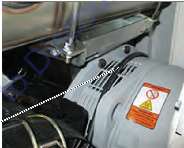
Figure 15 - Harness Routed Over Generator
