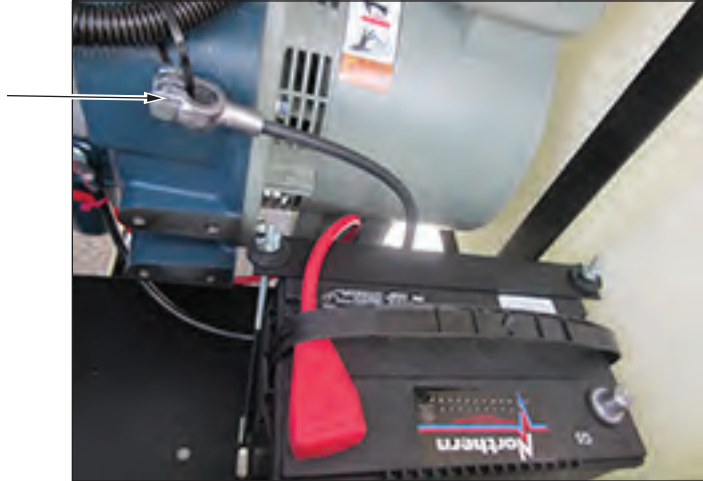
Figure 2 - Negative Battery Cable, Secured Away from Battery
