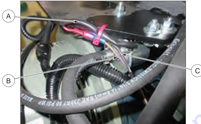
Figure 3 - Fuel Pump Wires
