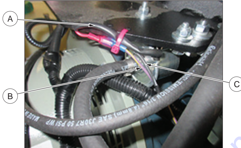
Figure 3 - Fuel Pump Wires
