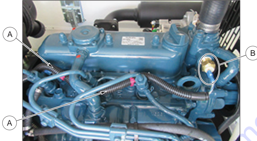
Figure 26 - Route Gray/Blue Wire to Coolant Temperature Switch
