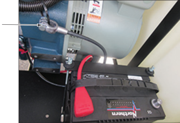
Figure 2 - Negative Battery Cable, Secured Away from Battery
