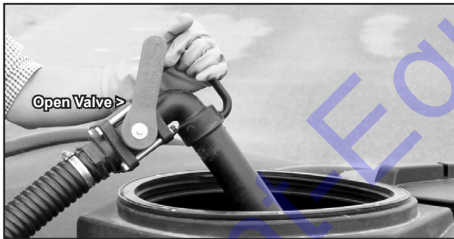
Figure B5 Valve Setting for Discharging Fluid
