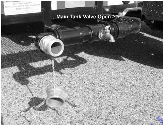
Figure C1 Main Tank Drain
