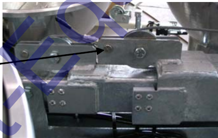
Figure 2. Cable Routed Through Pulley
