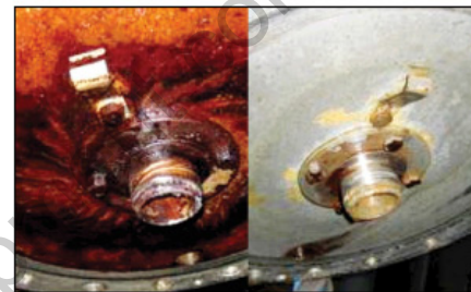
Vessel cover contaminated
