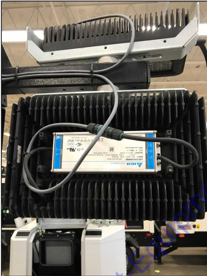
Trime wires to lights are simplified.
