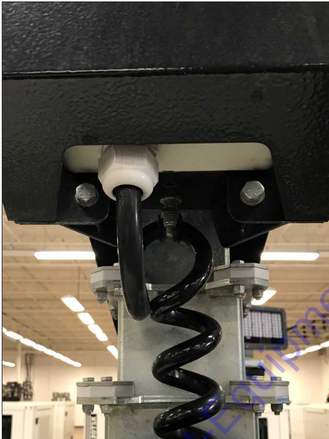
Trime wires protected by support so no pulling occurs.
