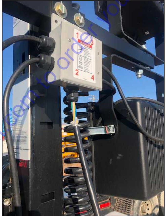
Competitor wires pull directly on electrical connection without support.
