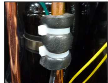
Figure 4: Thermistor attached to the refrigerant line.
