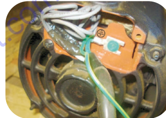
Grounding point in the engine.
