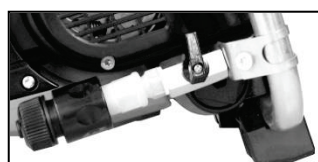
water supply closed (valve lever across)
