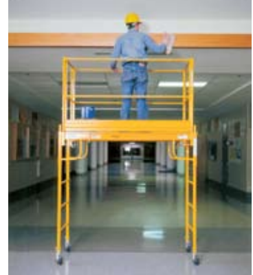
0127-006-1 shown in a maintenance application.
