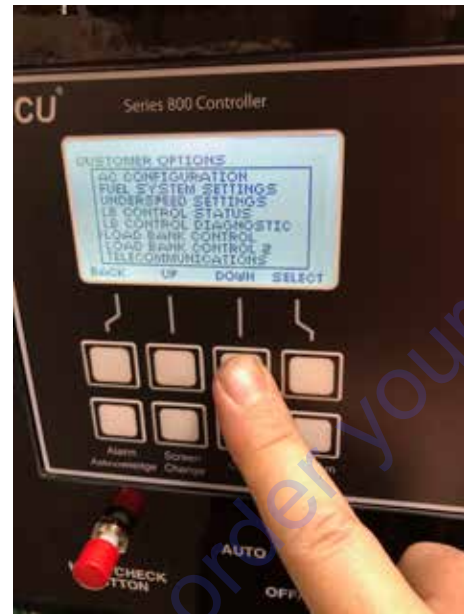
Figure 24. Load Bank Control
