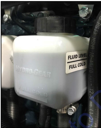
Hydro Pump Reservoir Tank
