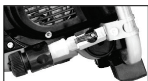
water supply opened (valve lever parallel)
