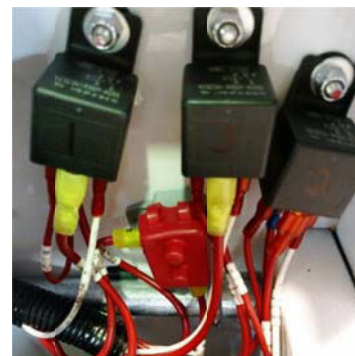
Figure 69: Circuit Breaker and Relays
