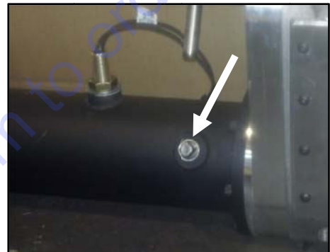
Figure 83: 3/8" Overflow Pipe Plug
