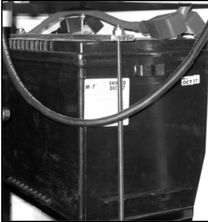
Figure 67: Battery and Brace
