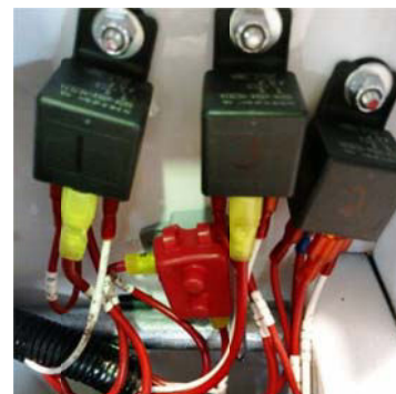
Figure 55: Circuit Breaker and Relays
