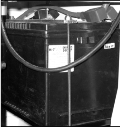
Figure 53: Battery and Brace
