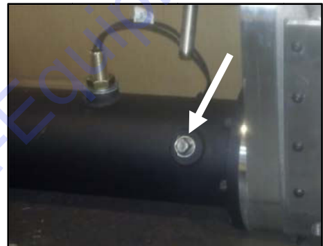
Figure 69: 3/8" Overflow Pipe Plug
