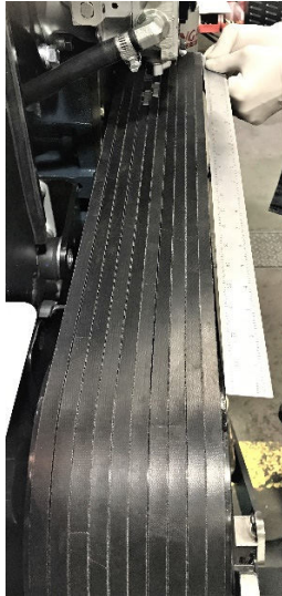
Jackshaft Sheave Alignment
