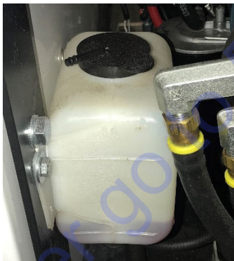
Coolant Recovery Tank
