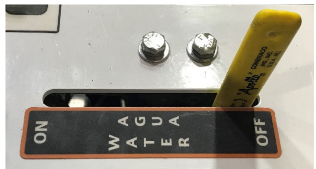
Water Valve - OFF
