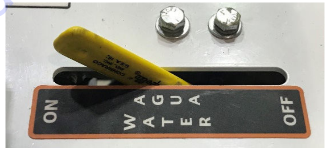
Water Valve - ON
