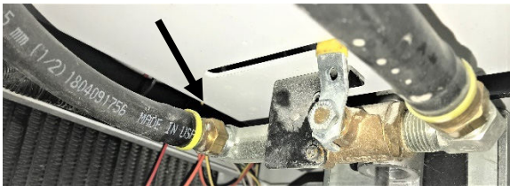
Water Valve Outlet Hose Connection
