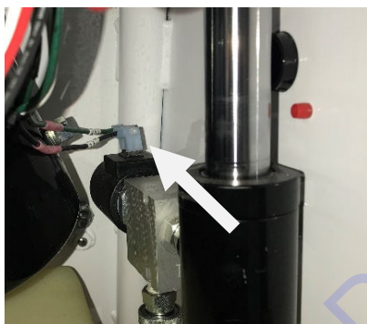
Solenoid Block Wires
