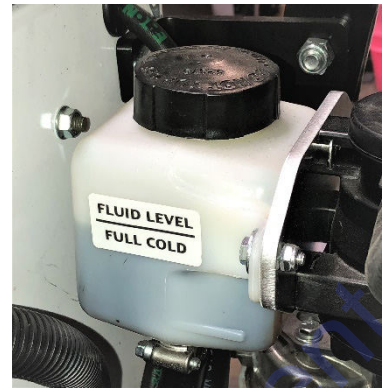
Hydro Pump Reservoir Tank
