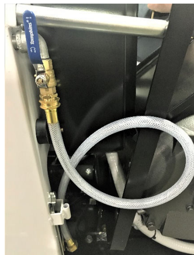
Right Water Flow Control Valve
