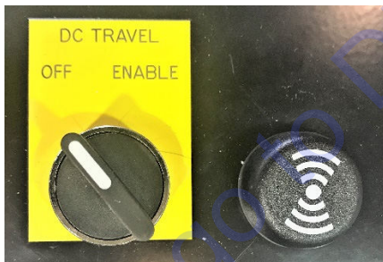
DC Travel Selector Switch and Alarm
