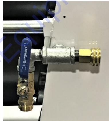
Water Supply Fitting and Left Water Flow Control Valve
