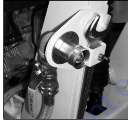
Figure 17: Water Supply Fitting
