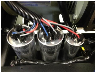
Chassis Mounted Potted Capacitors
