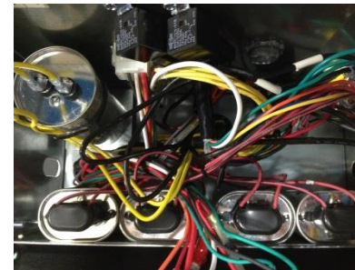
Box Mounted Open Terminal Capacitors
