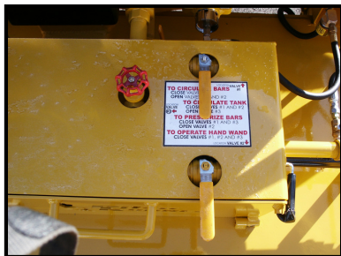
Pump Box Controls
