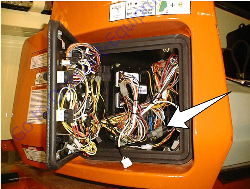
GROUND CONTROL CONNECTION
