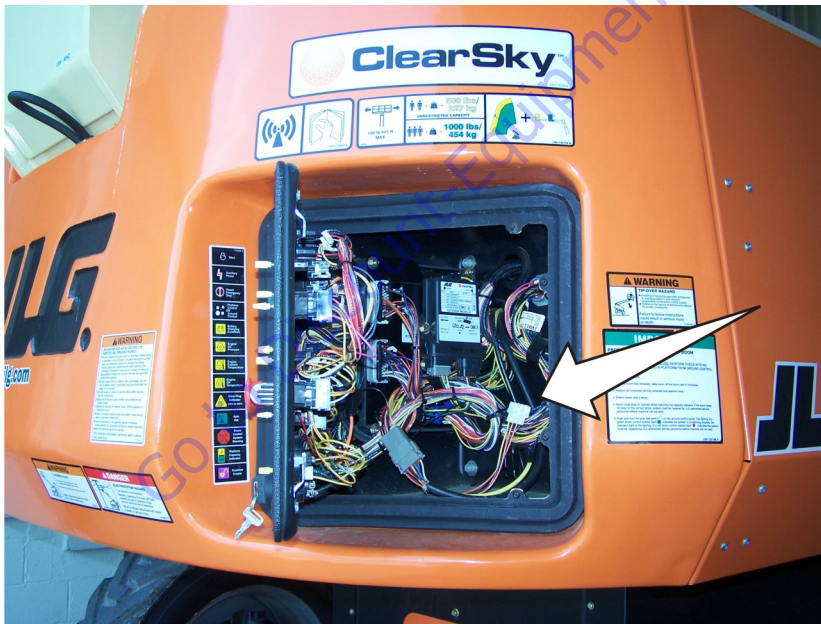
GROUND CONTROL CONNECTION
