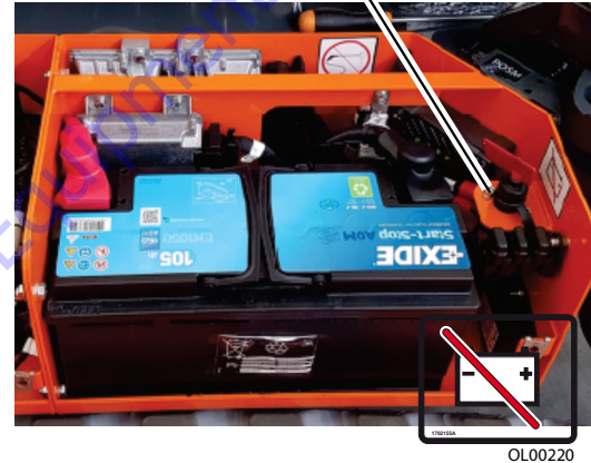
BATTERY DISCONNECT SWITCH - DIESEL/AC-ELECTRIC
