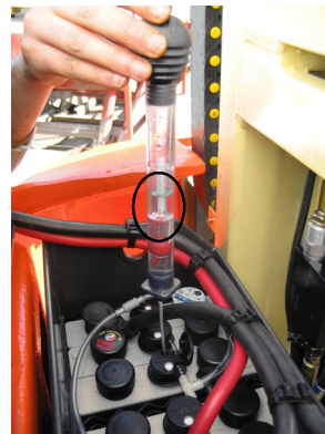
Figure 8-4. Measuring Electrolyte Specific Gravity
