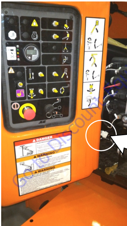
GROUND CONTROL CONNECTION
