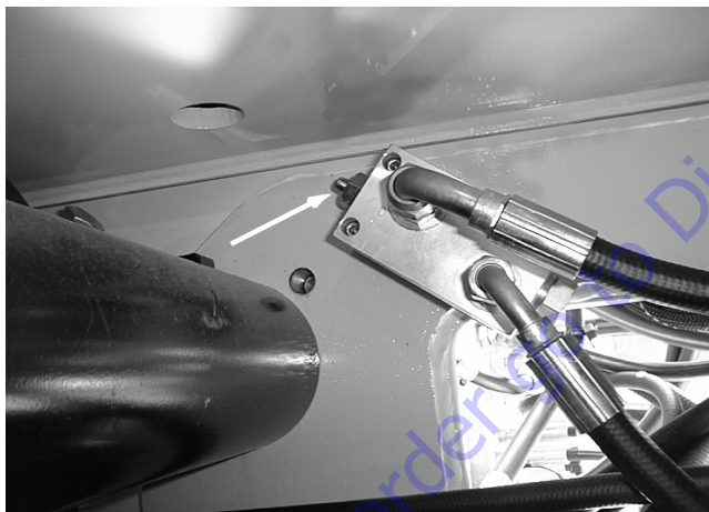
Figure 2-3. Tower Boom Vertical Limit Switch
