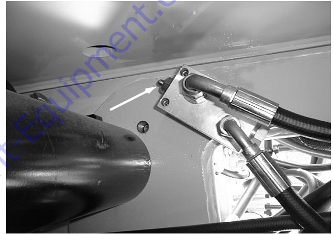
Figure 2-5. Tower Boom Vertical Limit Switch
