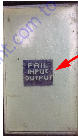
ELECTRIC CONNECTION ANOMALY IN PROGRESS
