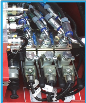
RIGHT SIDE GROUND VALVEBLOCK (10)
